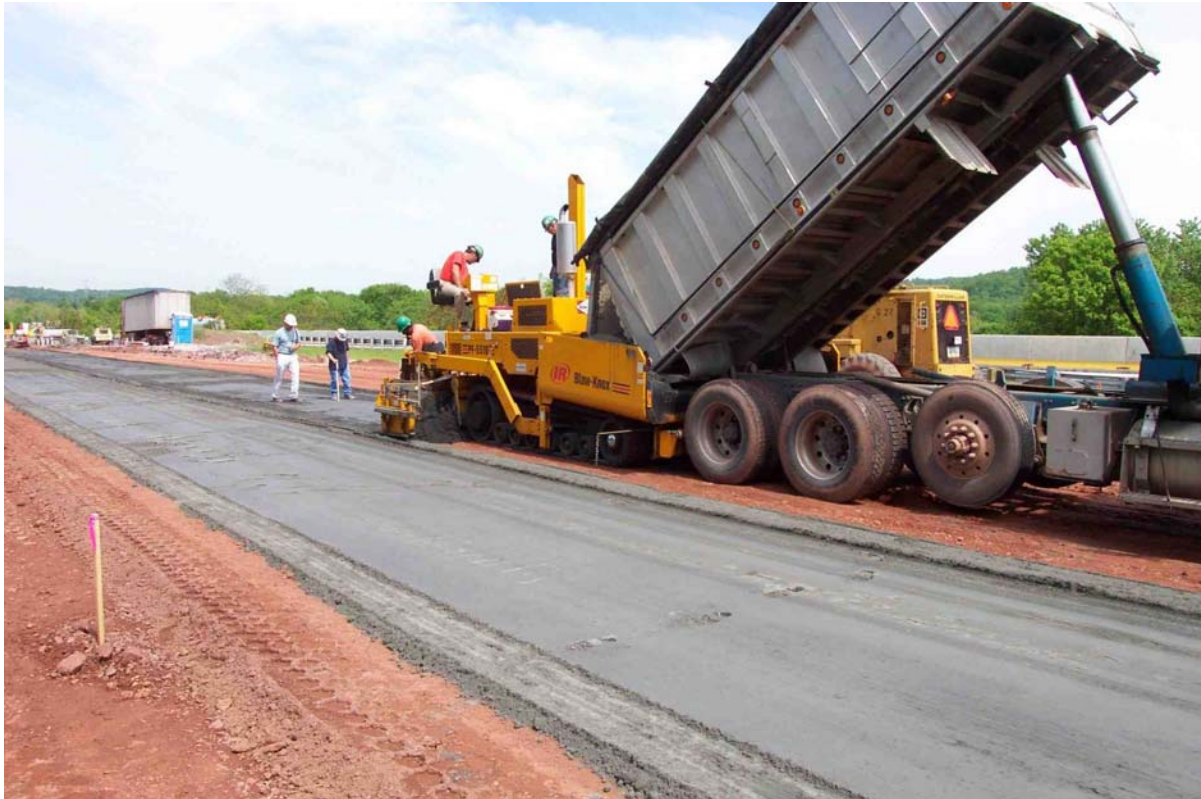
Figure 2: Moisture-conditioned fly ash from the PP&L Brunner's Island Power Plant being applied at 6% by dry weight soil on PennDOT SR-283.
