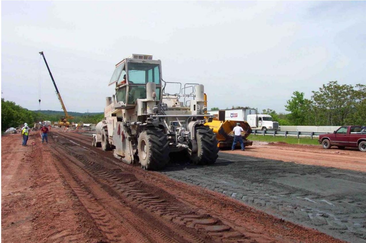
Figure 3: On PennDOT SR-283, a “road reclaimer” mixes moist-conditioned fly ash from Brunner Island, PP&L plant near Harrisburg, PA, to a depth of 12 inches. Lime had been similarly added on the previous day.
